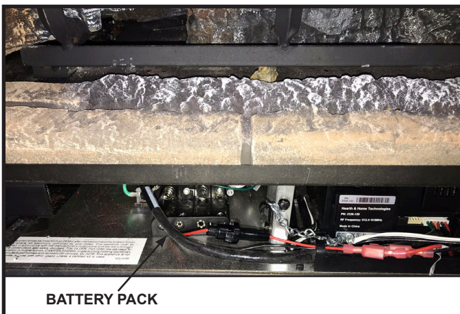
Figure 3.8 Battery Pack Installed
