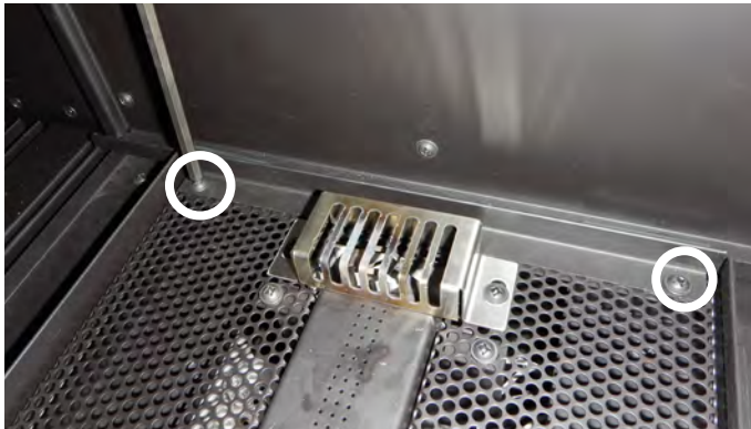
Figure 107. Pilot end of burner tray.
