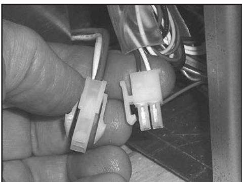
Figure 14: Disconnecting Standing Pilot Switch.
